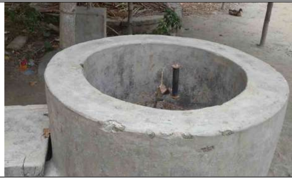
Bio-gas plant installation under MBSK SEP Project
